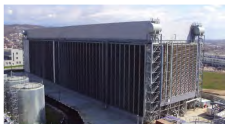
2 x 180 MW CCGP Adler, Russia, 2013 Induced draft steel structure dry cooling tower with supplementary spraying
