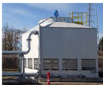
Wet cooling tower, Polgár W2E plant, Hungary
