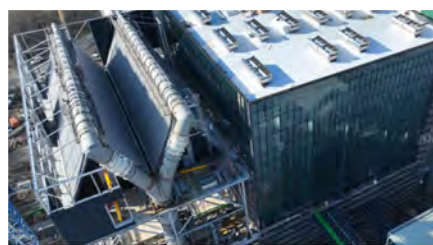
Waste to Energy Plant Warsaw, Poland, 2021 Direct air cooled condenser, single row heat exchangers
