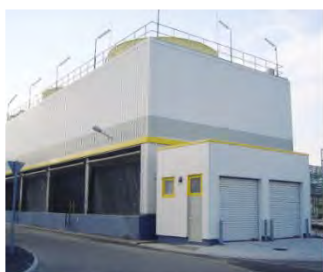
Wet cooling tower, BorsodChem, Chlorine Plant, Hungary
