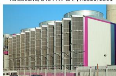
Induced draft steel structure dry cooling tower Tereshkovo, 340 MW CHP, Russia, 2011
