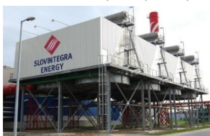
Direct air cooled condenser, single row, all aluminum heat exchanger Levice CCGT CHP Plant, 80 MW, Slovakia, 2007
